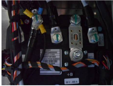
Fig. 10.8 – Controller power line protection
